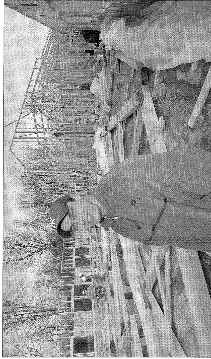
Jeff Mehrlige, executive director of Camp Kern, stands near building construction at the camp's main location a few year's ago. The camp — part of YMCA of Greater Dayton — has continued growing its main location, but will also open its first satellite camp in Greene County in 2011.
